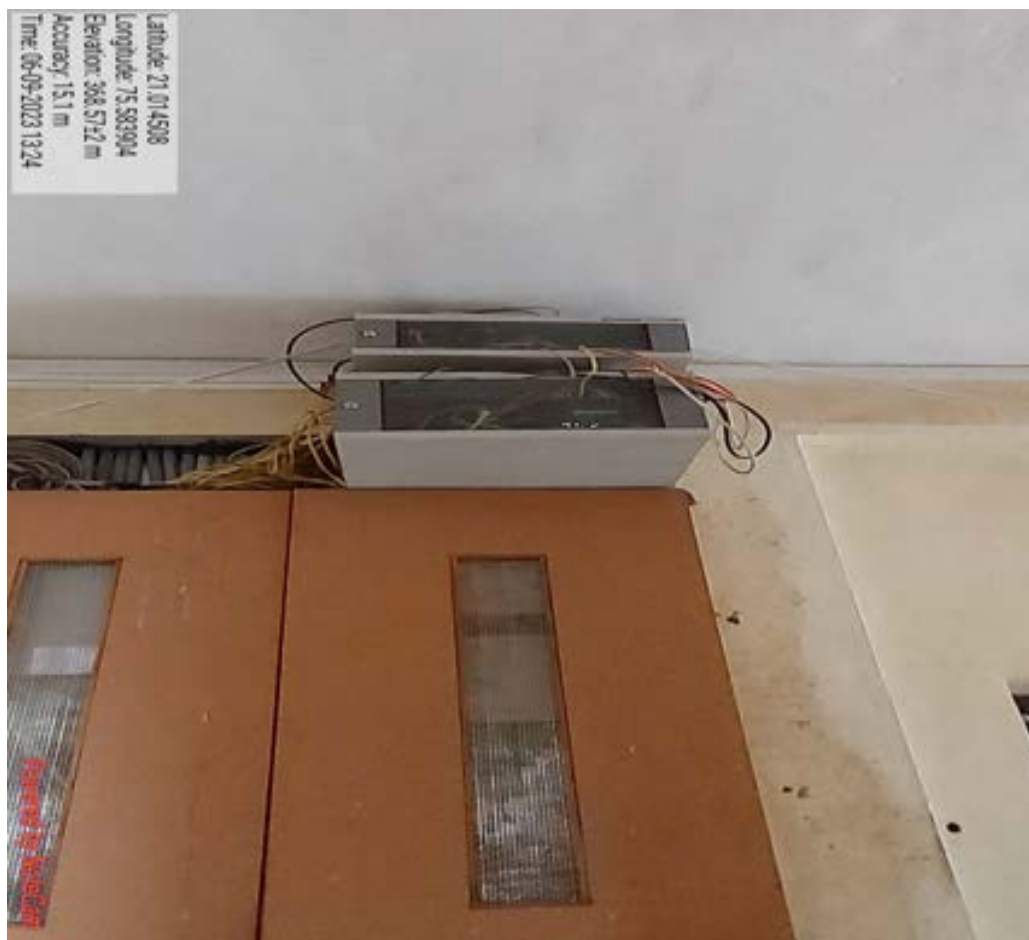
9. LAN FACILITY INSTALLATION
